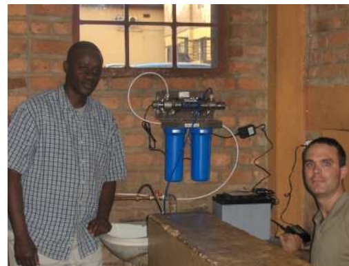
This water purifier was installed at the Gakinjoro Church in Kigali. This is 1 of 5 systems that we have installed in Rwanda so thousands of people will no longer have to choose between dehydration or disease.
